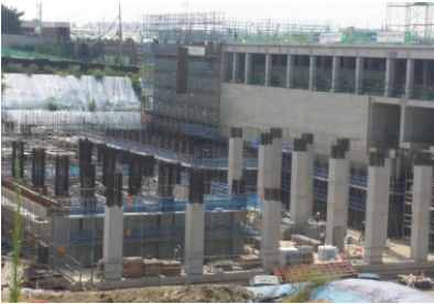
SEONAM WWTP | 190 MGD Comissioning Jan 2020
